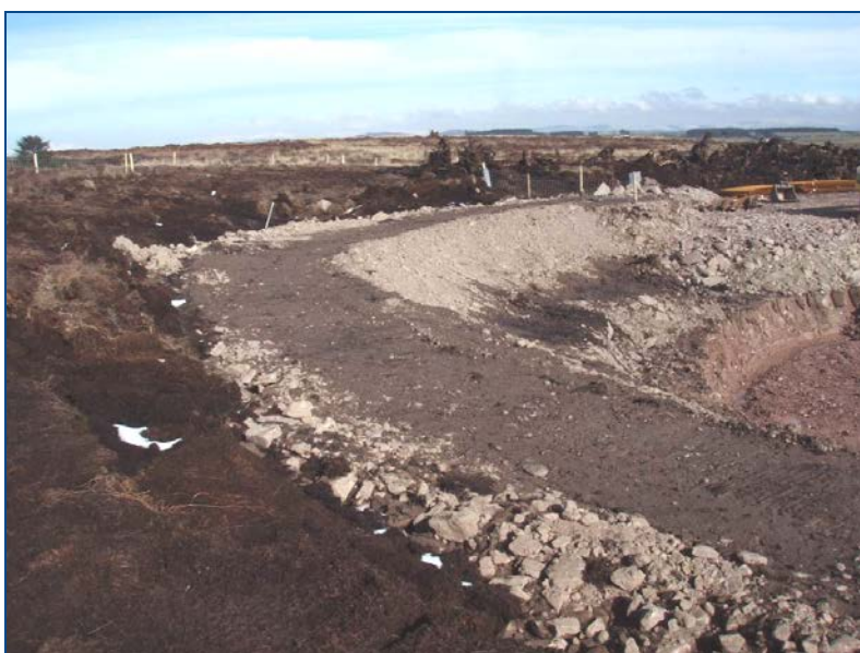
Figure 14.7: Rockfill Berm Around an Area of Deep Peat at an ESB Wind Farm
